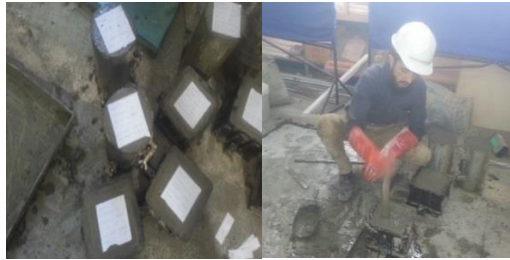
Fig. 6 Pouring concrete into the mold and freshly made samples with an information sheet
